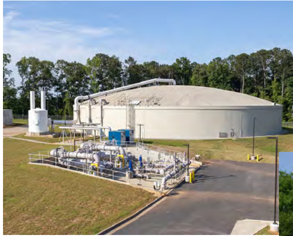
Water Treatment Facility
